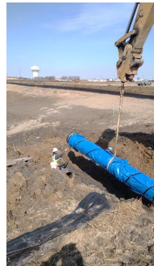
Twin 24" Storm Pipes that Connect the two Detention Basins
